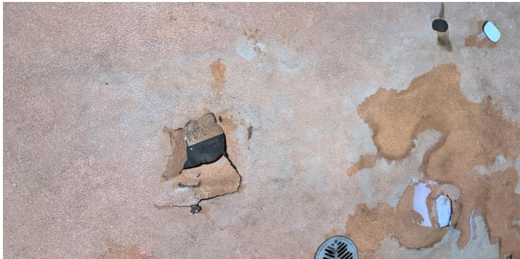
Figure 5: Bathroom floor at AACAP house in Pukatja. Image: Liam Greal
